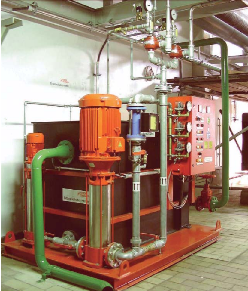
Pump set with storage container
